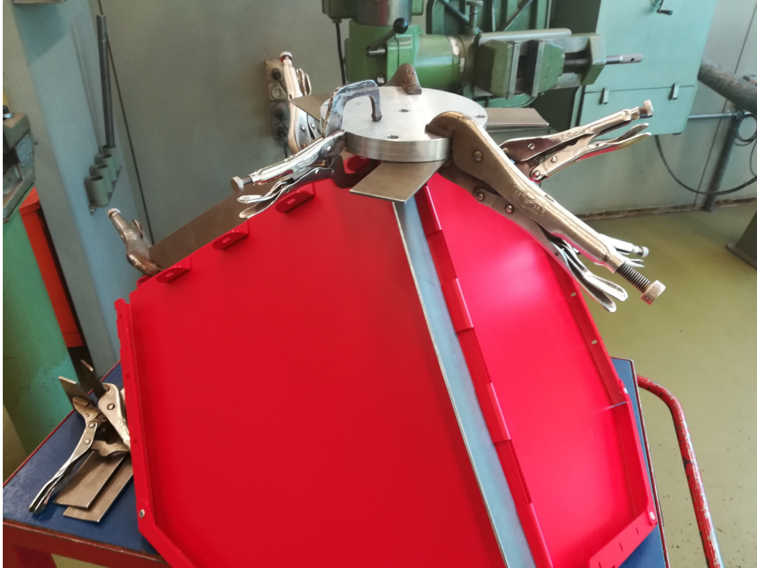
Figure A.16: Orienting and fixing the steel plates for the reflector mount to see if the angles are right and set position for wholes to connect the lashes with screws and nuts
