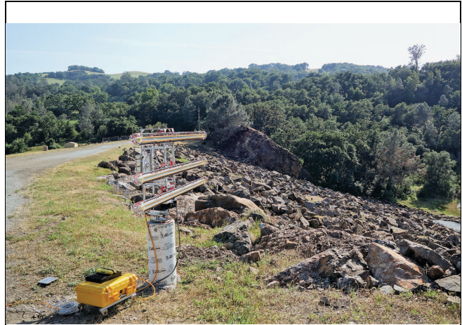
Figure 4: GPRI-II located at Pier B. Note the large rectangular silicate block close to fault plane just below the dam crest.
