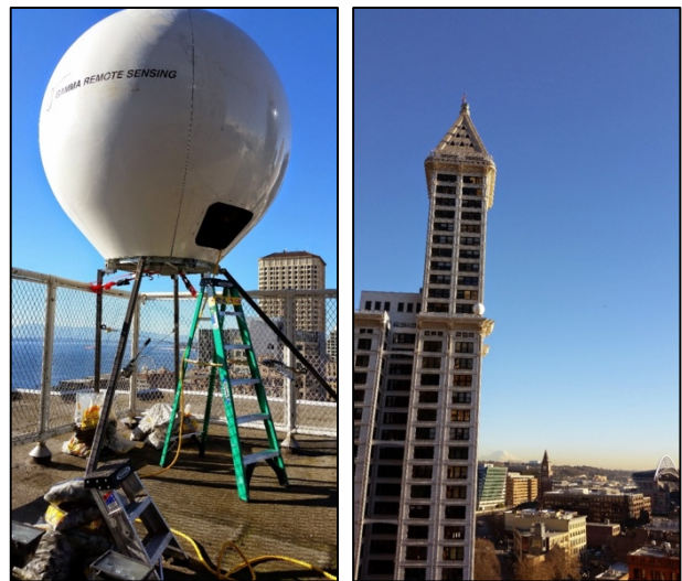
Figure 1 Deployment of the radar interferometer on the Smith Tower above Pioneer Square in Seattle
