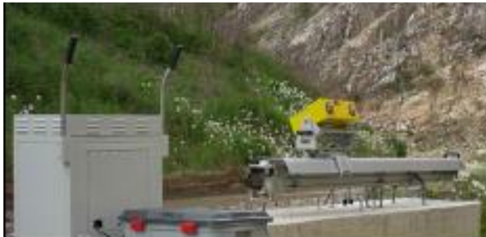
Figure 2.3. TRI, named IBIS-L, installed on a concrete foundation and used by Alba et al. (2008).
