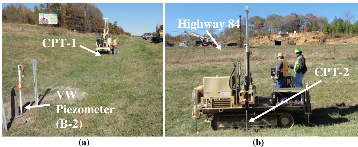
Figure 4.41. a) Cone penetrometer test being performed at the CPT-1 location, and b) cone penetrometer rig conducting the test at CPT-2 location.
