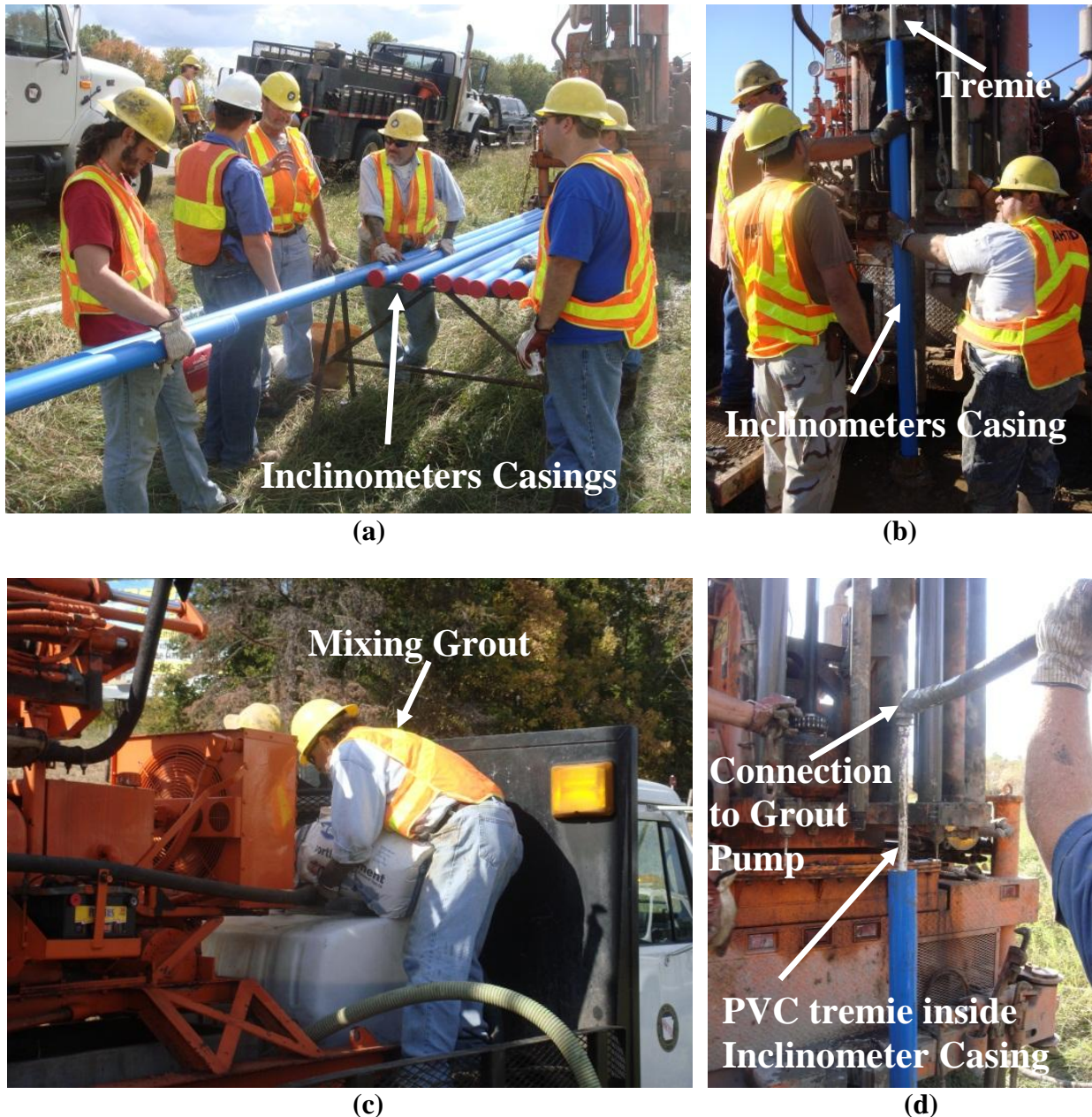
Figure 4.36. a) Sections of inclinometer casing, b) installation of inclinometer casing, c) preparing grout mix, and d) grout connection between tremie and grout pump.
