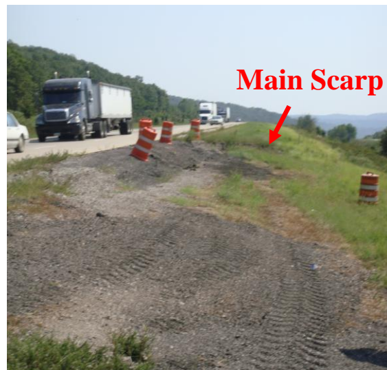
Figure 3.7. Traffic passing next to the main scarp in calibration site near Chester, Arkansas.
